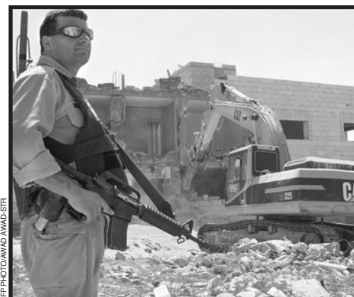
An Israeli policeman stands guard as a Caterpillar bulldozer demolishes a Palestinian home in East Jerusalem.
