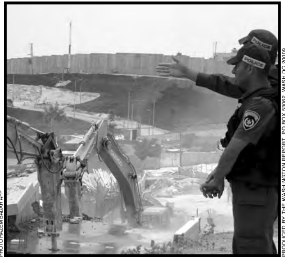
PHOTO HAZEM BADAR AFP PRODUCED BY THE WASHINGTON REPORT, PO BOX 53062, WASH DC 20009 Israeli policemen stand guard as a bulldozer demolishes a Palestinian home in the shadow of Israel's apartheid wall on the outskirts of Jerusalem on July 5, 2005.
