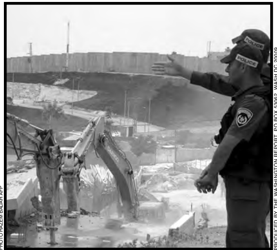
PHOTO HAZEM BADAR AFP PRODUCED BY THE WASHINGTON REPORT, PO BOX 53062, WASH DC 20009 Israeli policemen stand guard as a bulldozer demolishes a Palestinian home in the shadow of Israel's apartheid wall on the outskirts of Jerusalem on July 5, 2005.
